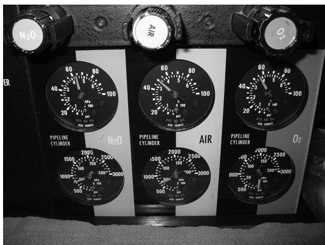
Fig. 3. The Narkomed 2B anesthesia machine medical gas pipeline gauges (Dräger Medical, Inc. Telford, PA) with the nitrous oxide line connected to the carbon dioxide wall gas outlet. Note that the nitrous oxide gauge is reading 62 psig, which is higher than one would expect if the line were connected correctly to the nitrous oxide wall outlet.
